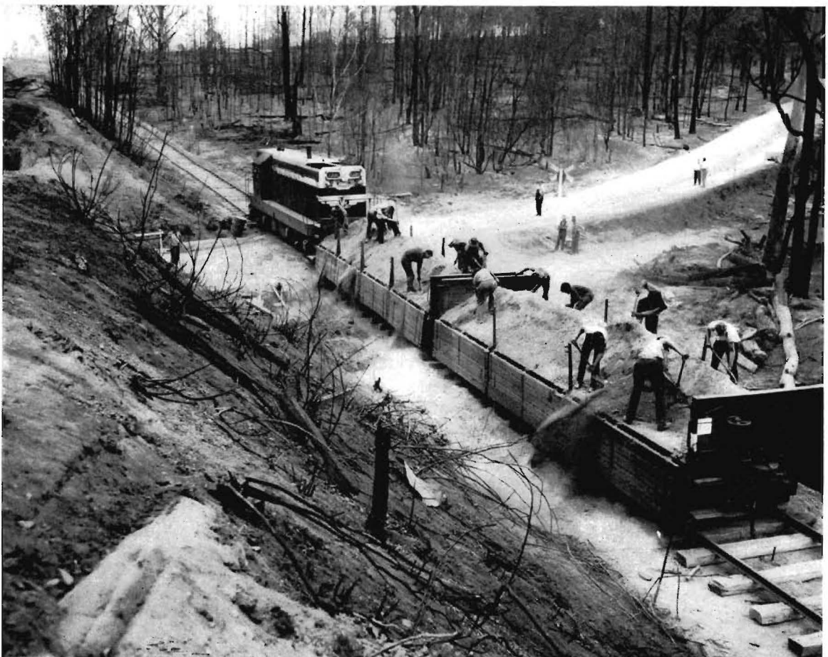
Construction of a temporary track deviation to replace a railway bridge destroyed by bushfires.
